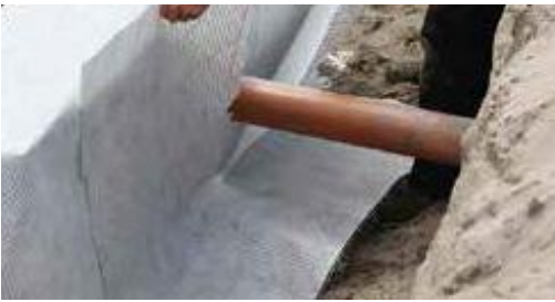
Use another piece of TPGeoGrid to make cover the cut. This cloth should overlap 1m left and 1m right of the utility.
