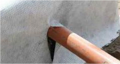
Make a straight cut in the TPGeoGrid around the TreeParker system up to the height of the utility.
